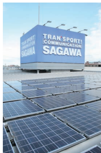
Solar power generation system
