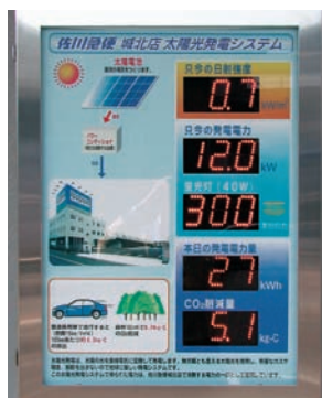
Solar power output display panel
